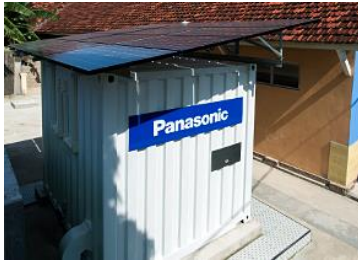
Compact photovoltaic storage system
