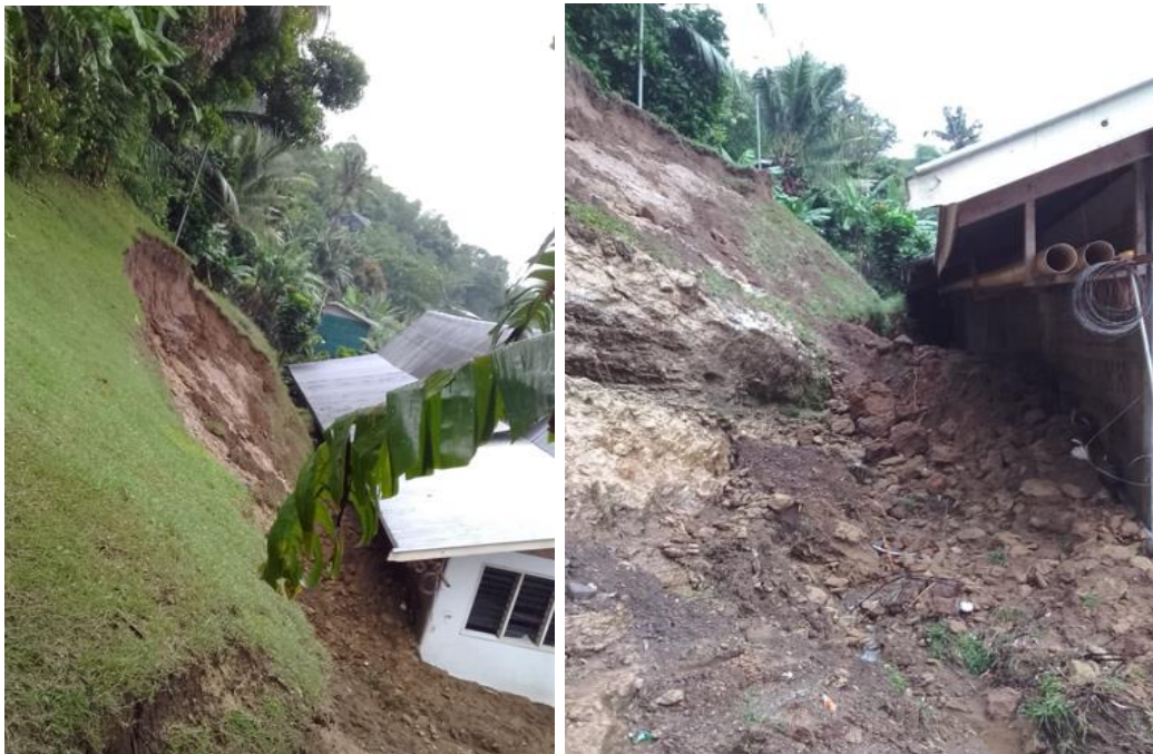
Landslide in Zone 27 following a heavy rainfall event on 11 Nov
