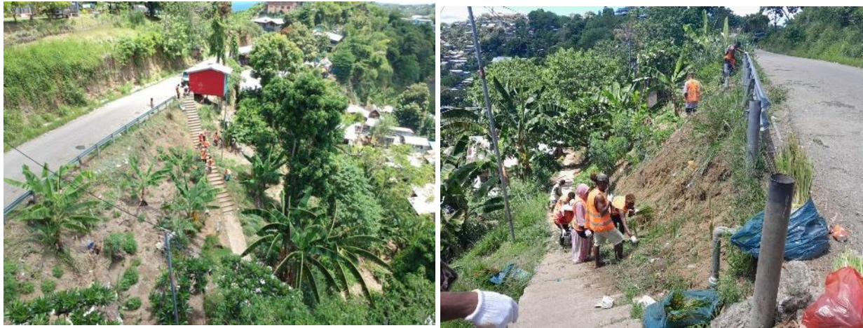
Clearing the track along Jacob's Ladder prior to planting vetiver grass to channel road runoff
