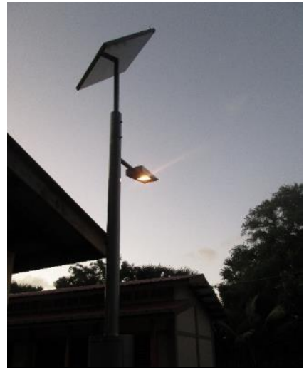
Solar lamp installed in the community centre compound.
