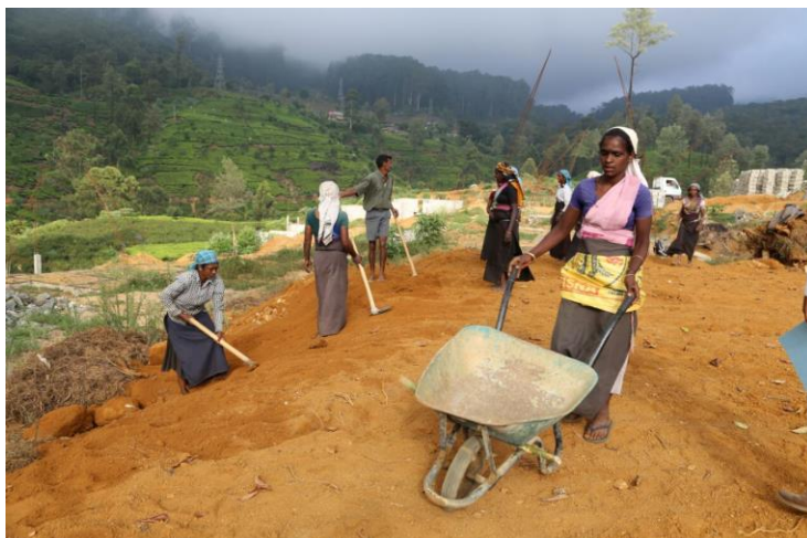
“Shramadana” activity by community members to clear and level the construction site.
