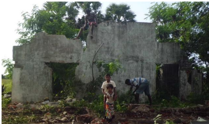
Mr.Anees’ damaged house in Puthuweli village.
