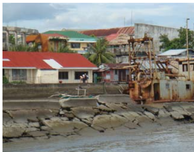
Damaged seawalls cannot mitigate the effects of storm surges and typhoons © UN-HABITAT/Yen Flores
