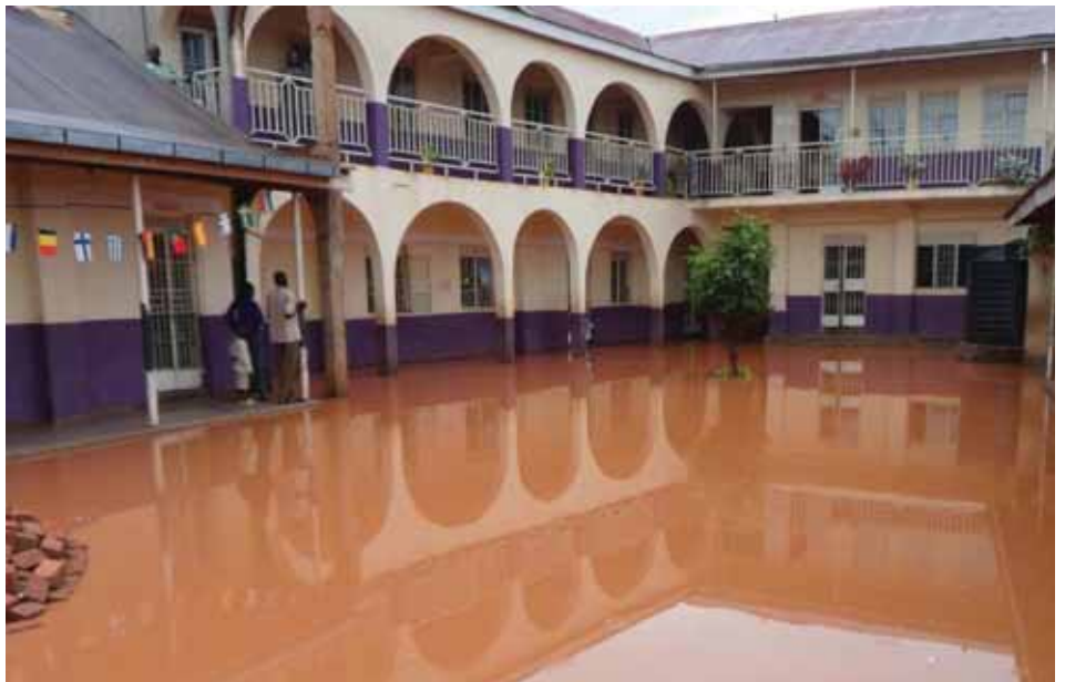
Flooded courtyard of Outspan Primary School in the Bwaise neighbourhood of Kampala, Uganda ©UN-Habitat
